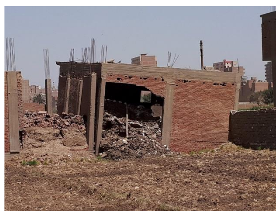
Figure 21: Collapsed house build on agricultural land in A3
